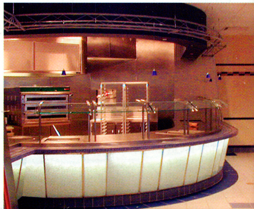
A conveyor deck oven, baker’s rack and thermal shelving units are in full view of customers at Reflections’ pizza station.
