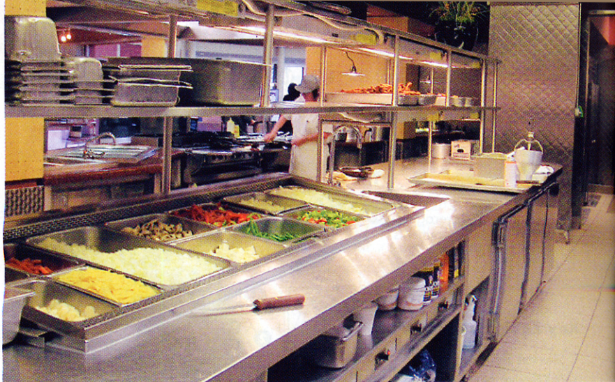
Holding wells for hot and cold foods and pass-through shelving were installed at the chef’s counter, which supports the Entrée and other stations.
